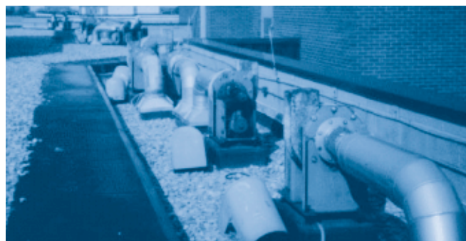
The centrifugal fans on this roof (with their housings removed) require monthly drive belt inspection, according to ANSI Z9.5 Standards. Mandatory maintenance adds costs and downtime, while possibly exposing workers to dangerous fumes.
