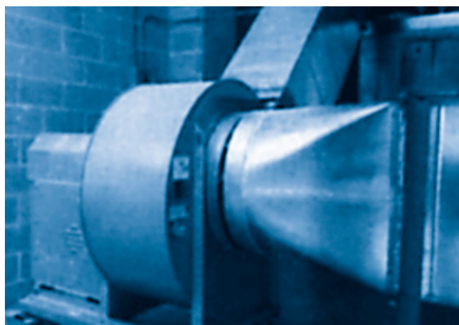
Centrifugal fans such as this complex installation are highly susceptible to inlet and outlet system effects, with corresponding losses in performance efficiency.
